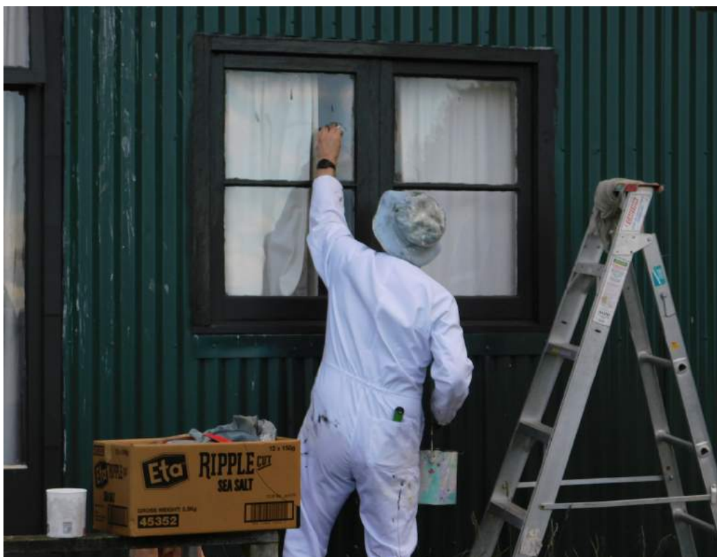
Chris wiping the paint off one of the windows. It should have been on the frame not the glass.
